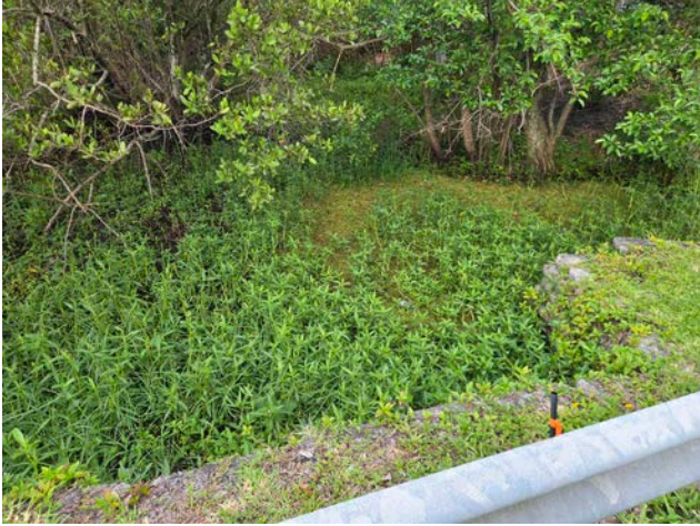
South side of Eagles Nest Drive — aquatic vegetation and duckweed backup at culvert outfall.
