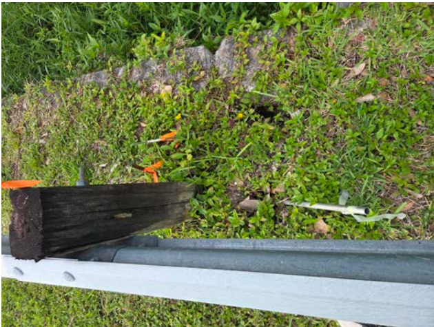
Close-up of void opening at guardrail post base — soil loss consistent with pipe failure below.
