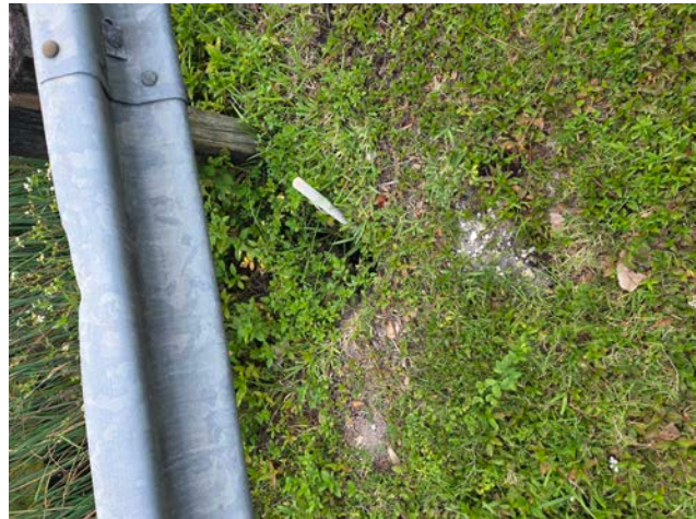
Additional ground collapse point near guardrail — lateral extent of subsidence along Eagles Nest Drive.
